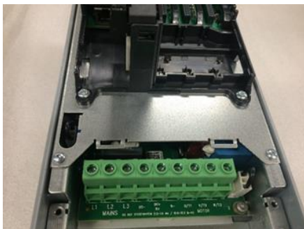
Figure 22 Frequency drive connections
